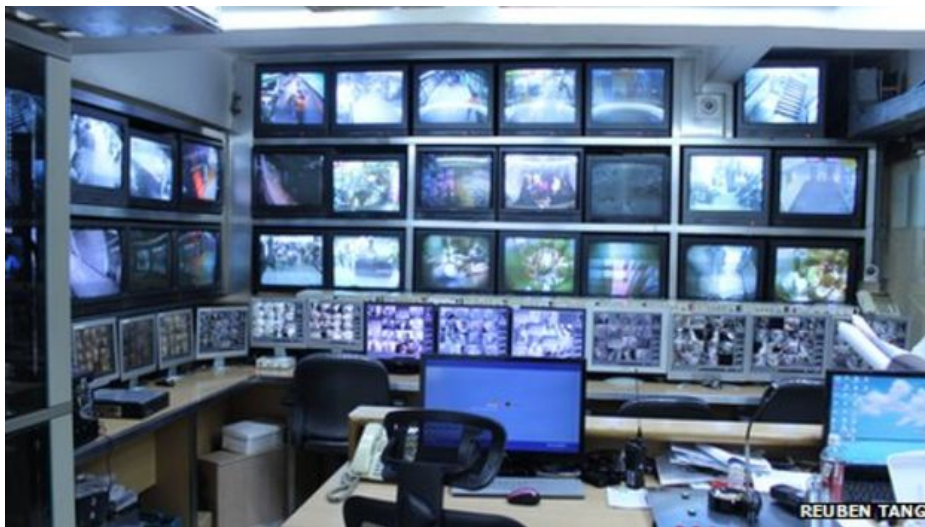
Its hundreds of CCTV cameras are monitored constantly
